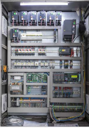
Kontrol Panosu Control Panel
