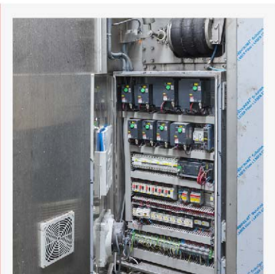
Kumanda Panosu Control Panel
